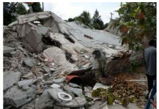
NVS after the earthquake— all that's left
